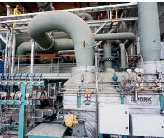
Wien Energie has assumed a pioneering role throughout Europe in decarbonizing district heating – not least thanks to projects such as the large-scale heat pump at ebswien.
