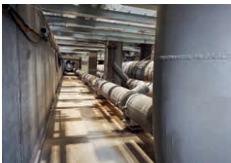
With a length of almost 50 meters, the pipe network runs in the plant’s basement, supplying the process with wastewater and coolant.
