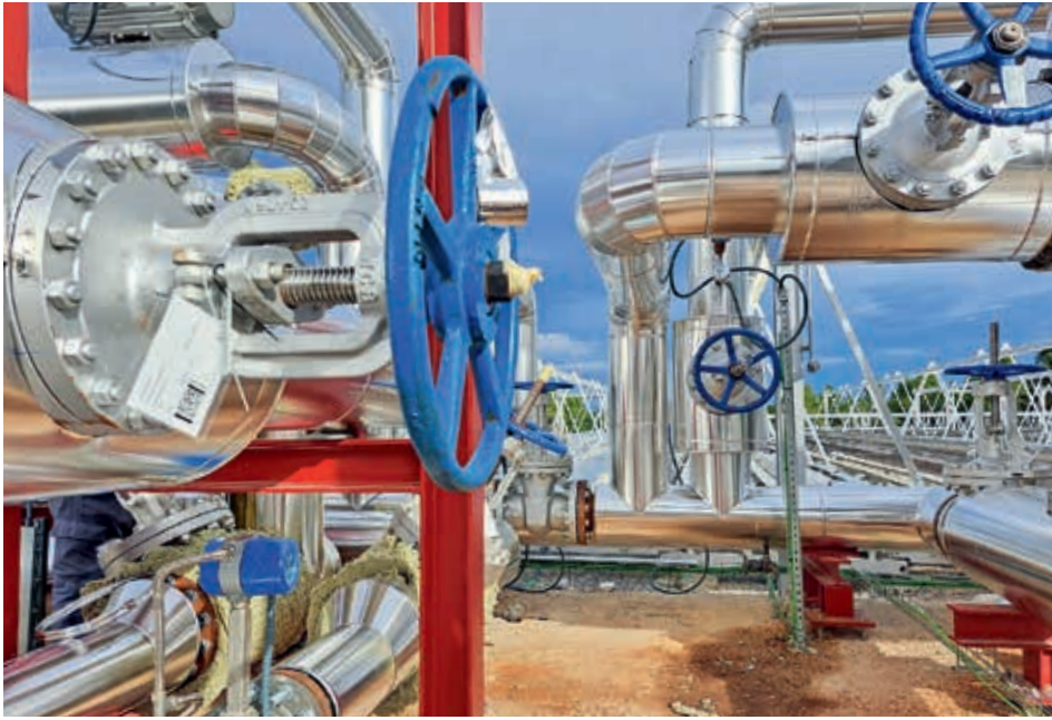
KLINGER valves are critical for shutting off the installation during maintenance.
